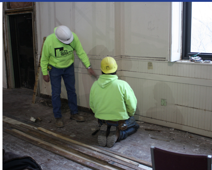
Construction crews had to be careful to know what was being restored and what was being replaced. (Top) Carl stands amid what will be the new circle drive entrance.
