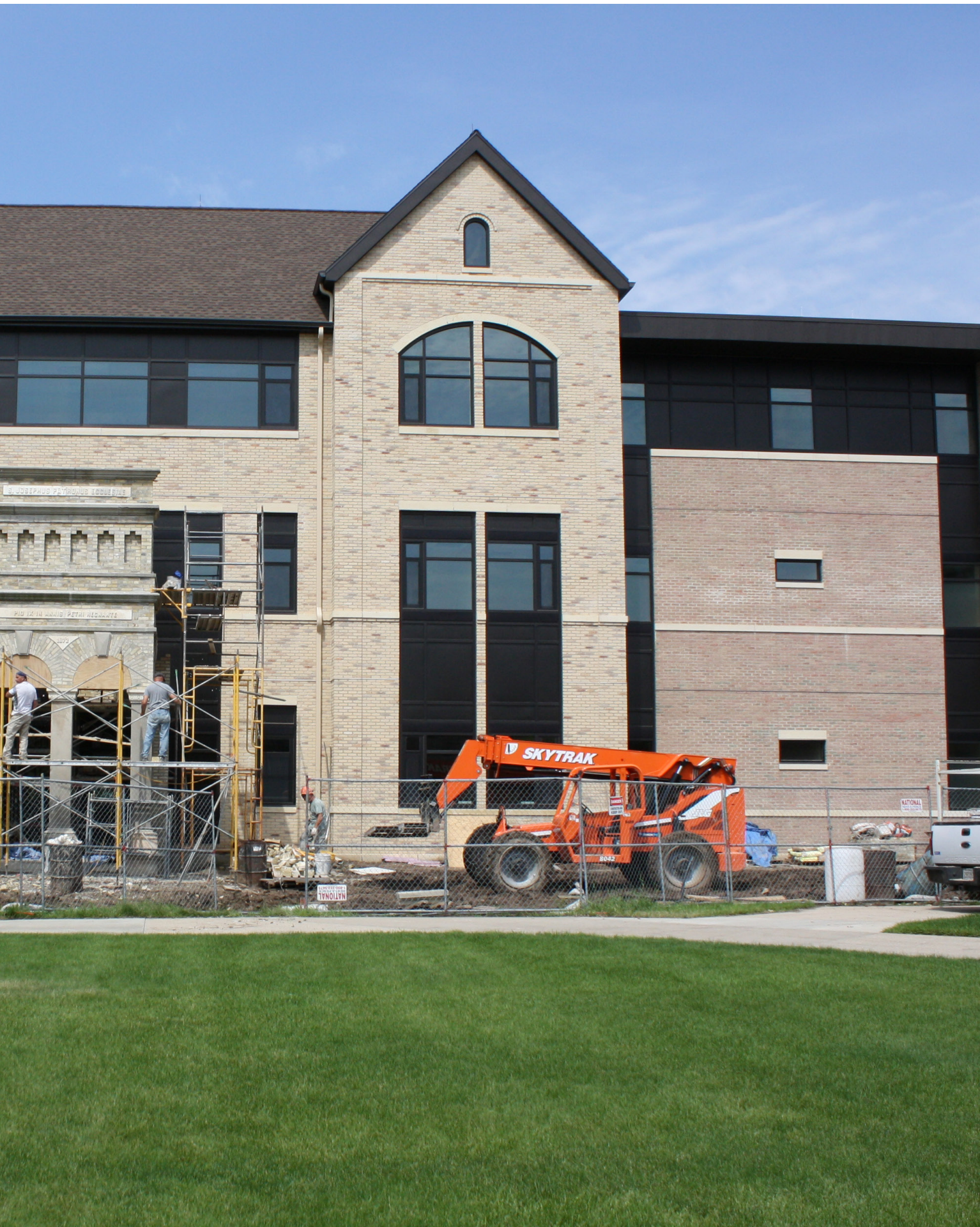
Masons reconstruct the portico from the old St. Joseph Hall brick by brick.
